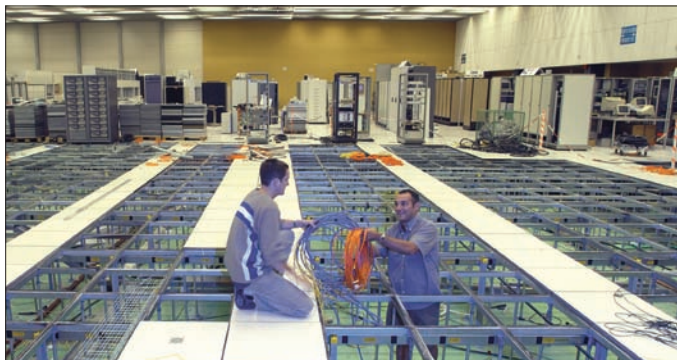
Renovation of the Computer Centre at CERN in July 2003. Half of the equipment of the large ground-floor room has been removed. A large-scale spring-cleaning operation took place before the renovation. Workers removed 15 km of cables that were no longer needed from the cavity floor for recycling, to prepare for PC farms.
